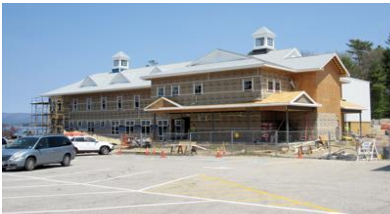
Construction on the 32,000-square-foot Marine Patrol building continues apace with a scheduled completion date in October. (Laconia Daily Sun Photo – Gail Ober)
